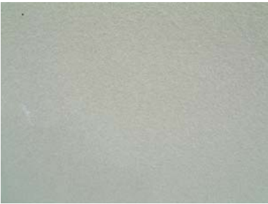
Smooth Finish – No surface defects
